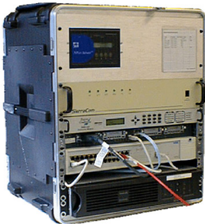
Figure 5: Indoor-Unit of the VSAT.
