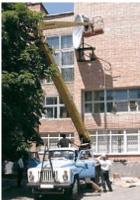
Installation in Russia
